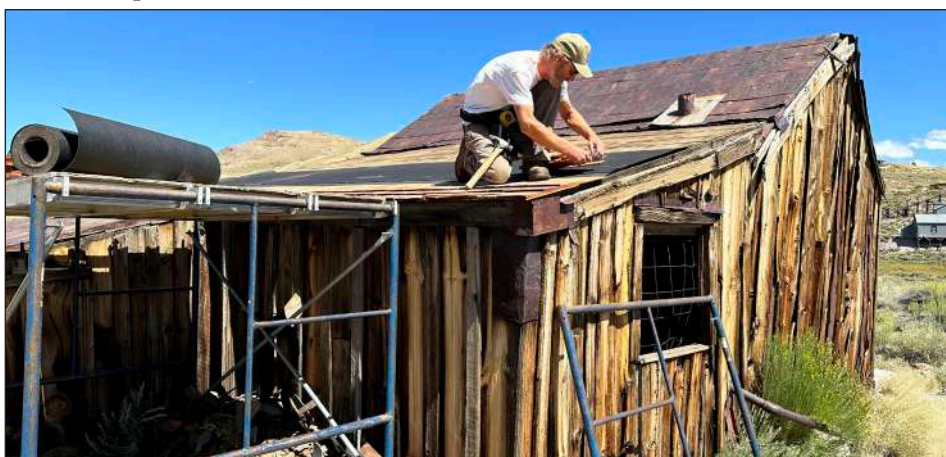
Eric Draper works on a roof in Summer 2023, following a winter of record snowfall.
