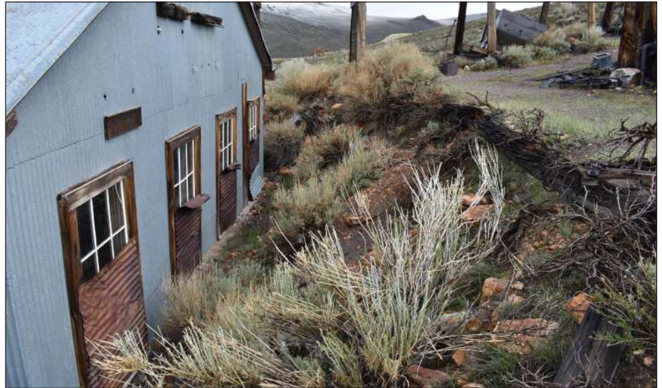
Bodie Foundation has launched a new fundraising project for the Stamp Mill. Work has started on erosion at the back of the building.
