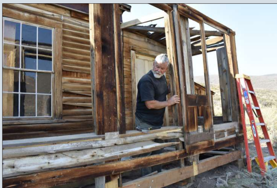
Bodie SHP Maintenance Worker I Kevin Russell works at the Tracy House in the north end of town. The front porch was shored up with a new beam to help stabilize the structure.
