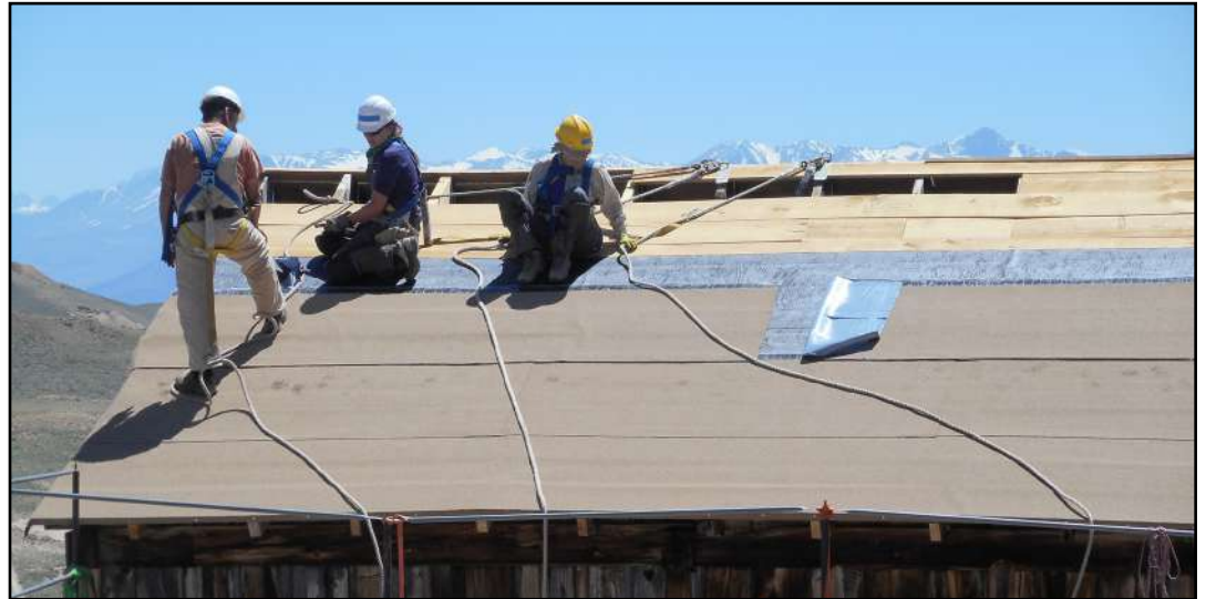
A trio of HistoriCorps volunteers at work on top of the Standard hoist building had a view of the Sierra Nevada during roof repair this summer. Photo by Brad Sturdivant
