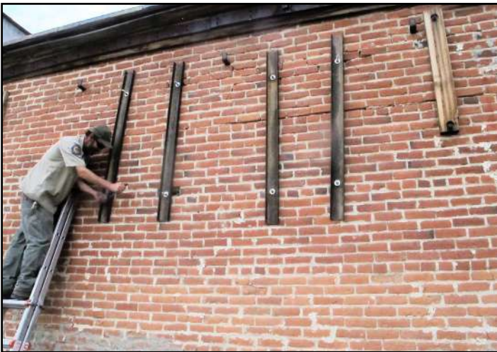
Park Maintenance Assistant Eric Draper lines up a metal bar with threaded bolts to re-align the brick and mortar on this earthquake-damaged wall. Photo by Katie Ogle
