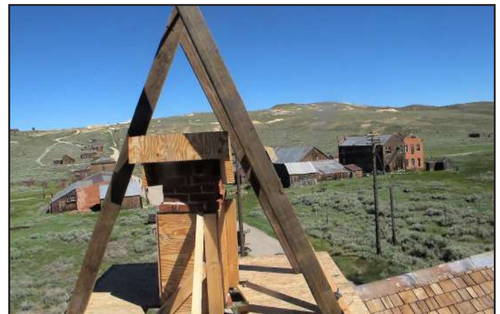
To repair the J.S. Cain house chimney, workers built a platform and clamped the chimney down with compression straps. They then put on an A-frame, lifted the chimney a couple of inches and put it back square. Photo by Paul Serna-Garcia
