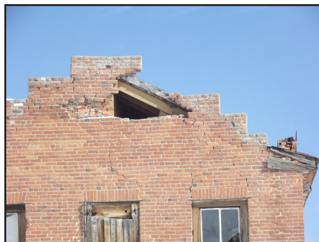
Powerful earthquakes in December 2016 shook open a hole on the west side of the DeChambeau Hotel. Photo by Brad Sturdivant
