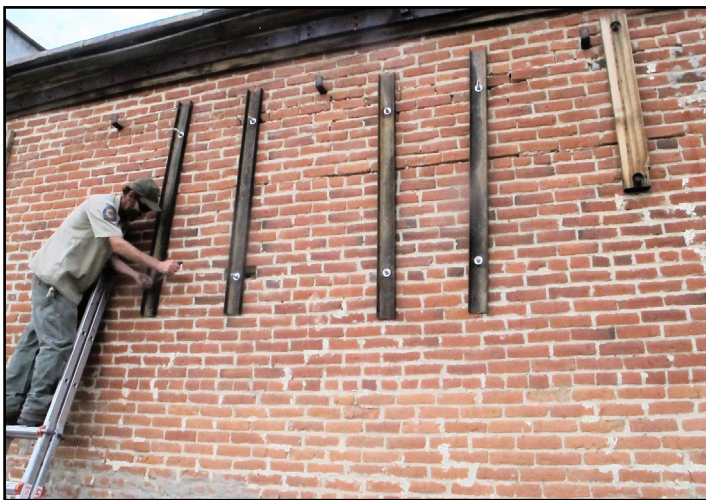
Park Maintenance Assistant Eric Draper lines up a metal bar with threaded bolts to re-align the brick and mortar on this earthquake-damaged wall. Photo by Katie Ogle
