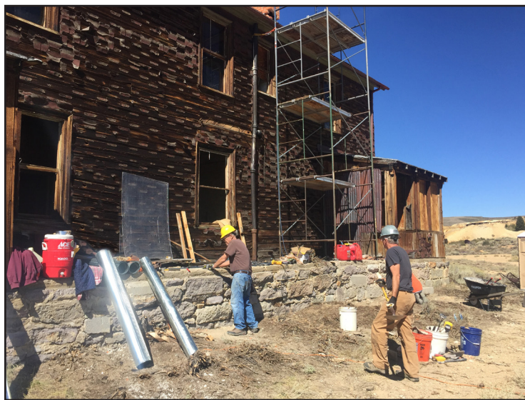
A crew from HistoriCorps, a nonprofit organization that provides skilled volunteers to preserve historic structures on public lands, works at the Bodie Railroad Office in September. Photo by Shayla Geissinger
