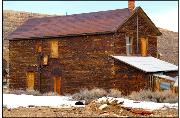
The rusted roof of the train depot office building (near water tower) is one of six arrested decay projects being funded by the Bodie Foundation. Bodie's original structures are under constant attack from the area's harsh climate. The goal is to keep the structures as they were when Bodie became a State Park in 1962.
